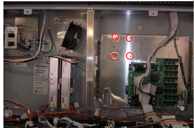
Location of tie wrap holders on a sign with a 12-channel daughter card.
