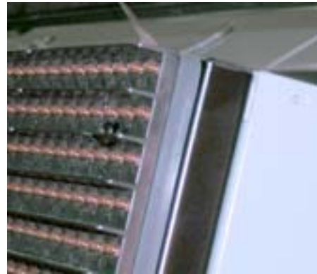
↑ Properly functioning driver board. No gap is visible.
